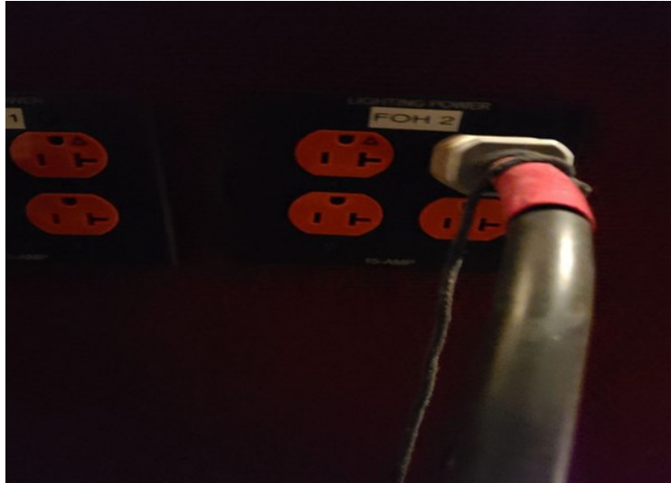
(2) 20 amp circuits at FOH Position
